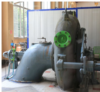
Turbine type Francis Phot. Samir Mahfoudi, Autr. Samir Mahfoudi IVR82_20117401210NUCA
