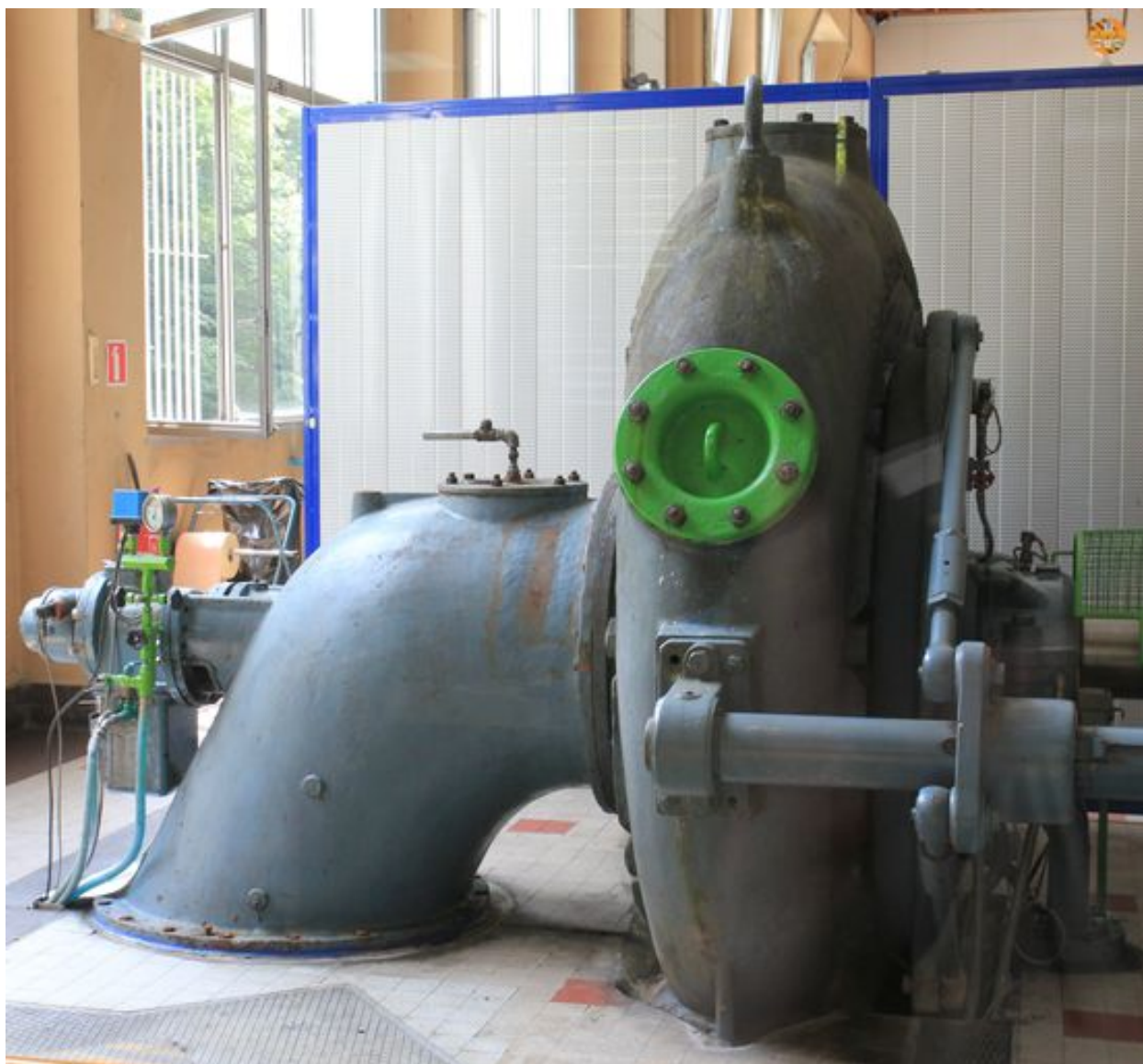
Turbine type Francis
