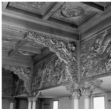
Consoles Phot. Didier Gourbin IVR82_20066902194X
