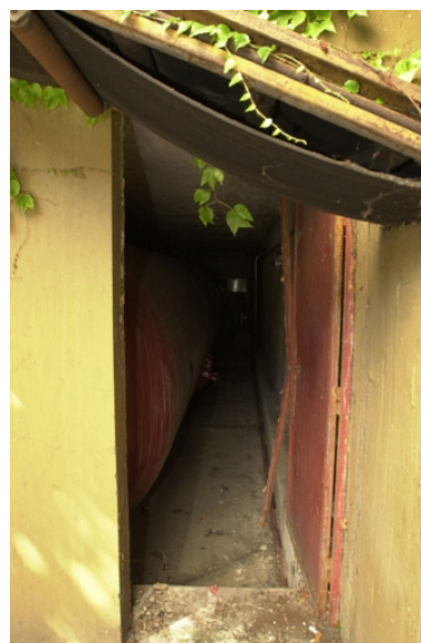
Emplacement cuve Phot. Nadine Halitim-Dubois IVR82_20036901951NUCA
